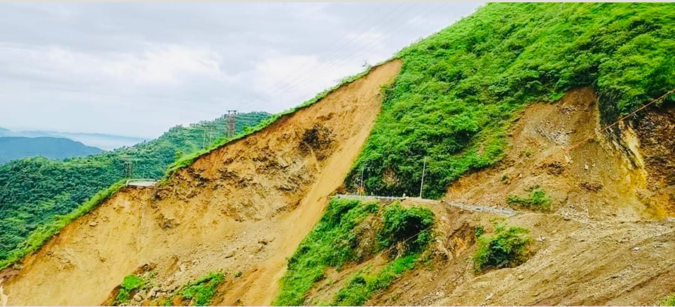
Commuters had a narrow escape when a stretch of national highway (NH) 707 was swept away in a landslide near Barwas in Kamrau tehsil of Sirmaur district on July 31, 2021.
