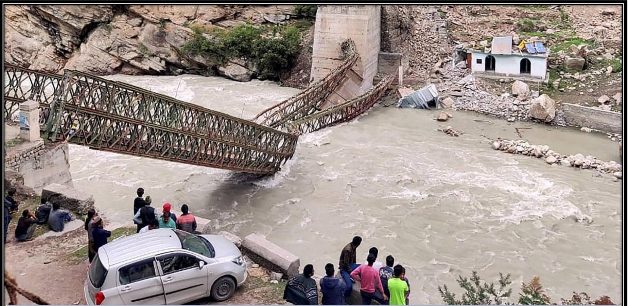
A bridge collapses after a massive landslide in Himachal Pradesh on Jul 25, 2021
